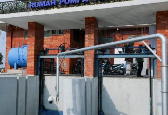
The Yos Sudarso Pump House is one of the locations where the Tide-Eye system has been implemented, supporting tidal flood control with real-time tide data.
