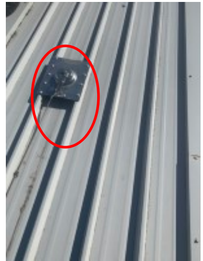
Roof area landing with 360 anchor & stop (Certification by Riverlands Roofing Status Current)
