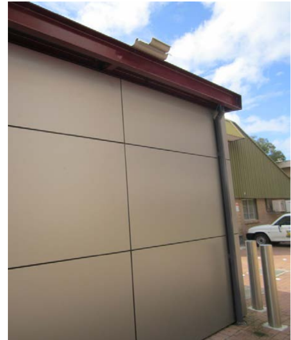
Ladder bracket on Western side
