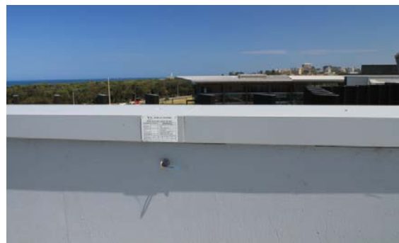
Anchor point to access landing
