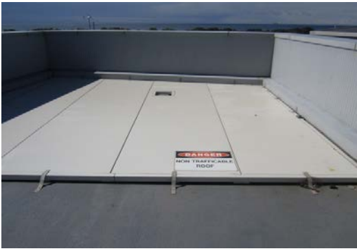
Skylight covering now enclosed - unsafe
