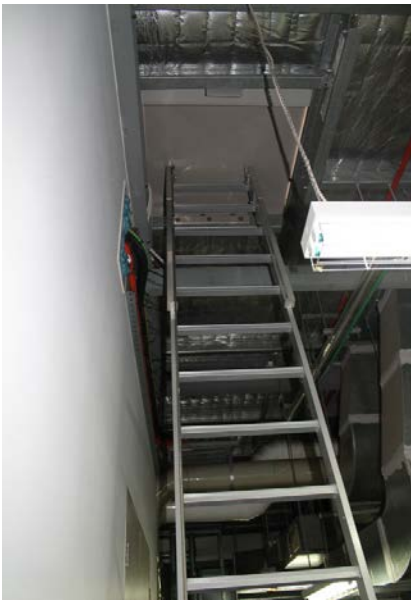
Ladder and hatch in plantroom to upper roof
