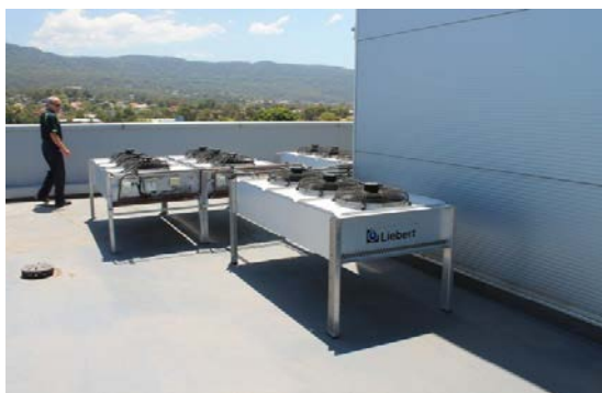
Air-conditioning units on south-west side
