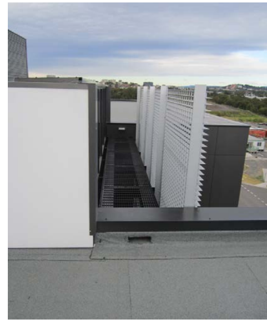
Window cleaning walkway on building exterior
