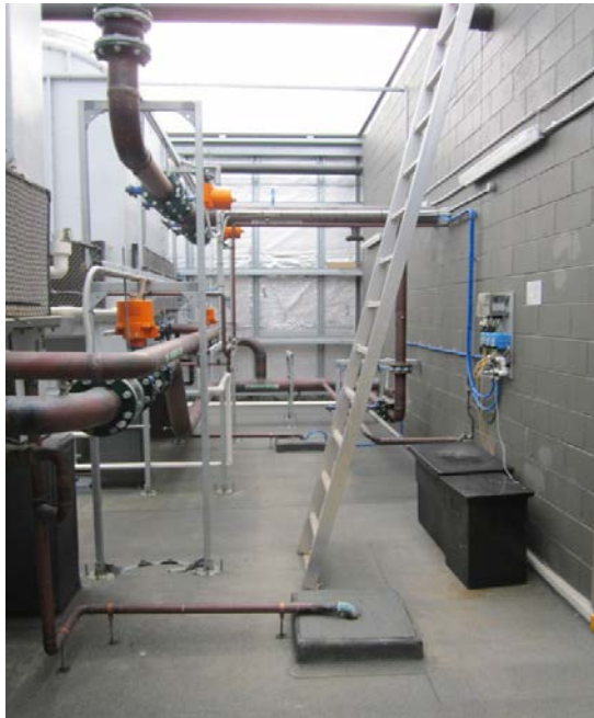
Airconditioning and ladder up to roof from western plantroom
