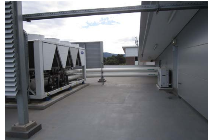
Airconditioning service area
