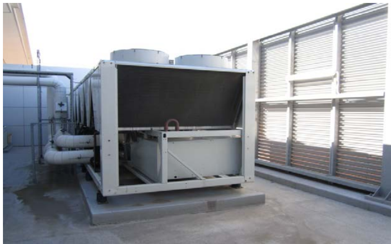
Enclosed area for air conditioning services
