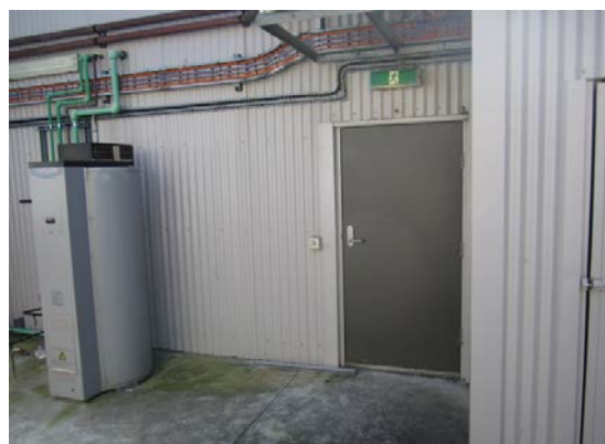
Access door to outside plantroom
