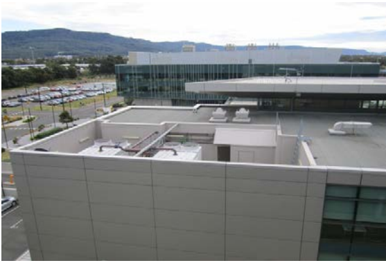
Exterior plantroom in SW corner
