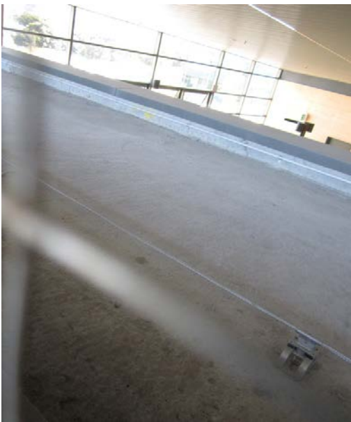
Interior horizontal lifeline above offices
