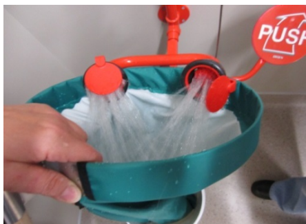
Figure 4 Testing Eyewash station
