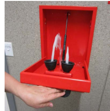
Figure 5 Eyewash station inspection
