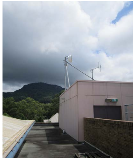
Microwave tower on plantroom roof
