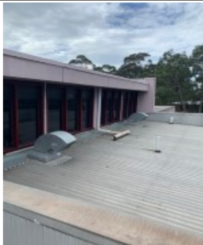
Main roof area with ducts
