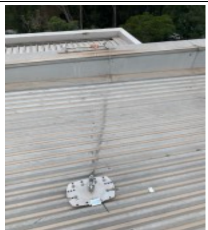
Upper roof area with anchor & strop (Certification by Riverlands Roofing Status Current)
