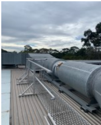
Main roof area with walkway, handrail leading from the roof access hatch and ducts
