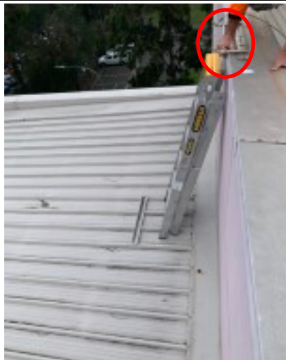
East roof with portable ladder access, ladder bracket Caution when climbing down the ladder user to be connected to the strop
