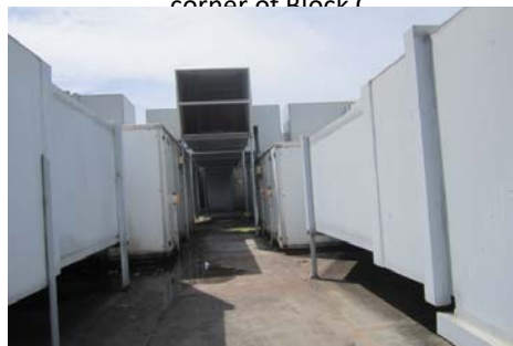
Looking up to access door in the main services area on Block C
