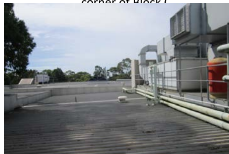
Handrail on the northern side of the main services area on Block C - looking east towards Block B
