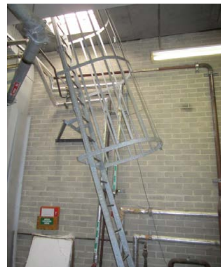
Ladder and hatch to access on Block A Caution - Low head clearance on access ladder.
