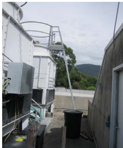
Ladder to cooling tower on Block B
