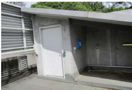
Roof access to enclosed services area in SW corner of Block C
