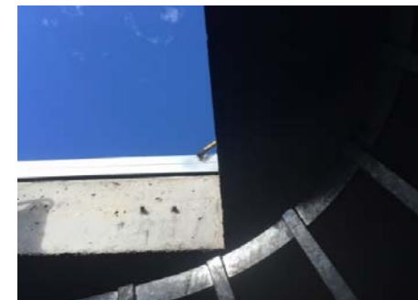
B39 low head clearance on ladder
