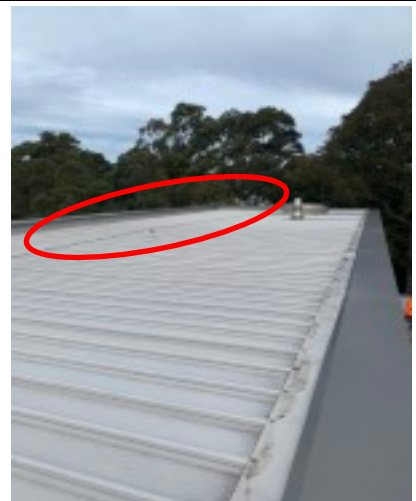
Upper roof area with vertic lifeline ( Certification by Riverlands Roofing Status Current )
