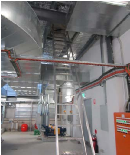
Ladder in plantroom
