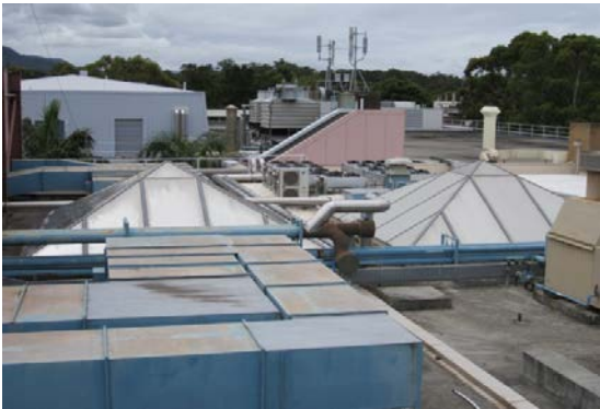
A/C vents and skylights
