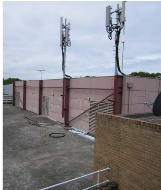
Telco Tower on Building 17 Roof
