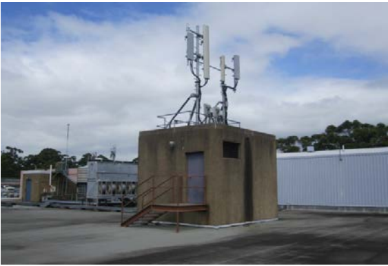
Telco Tower on Building 17 Roof - Northern side
