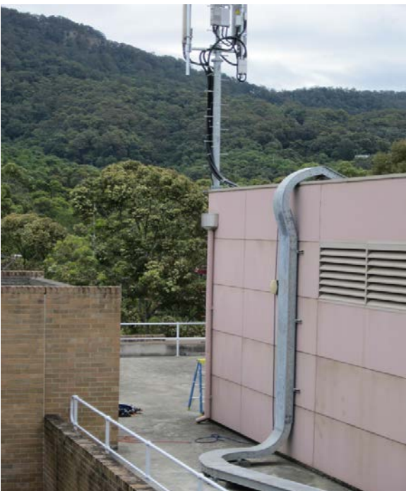
Telco Tower on Building 17 Roof - west
