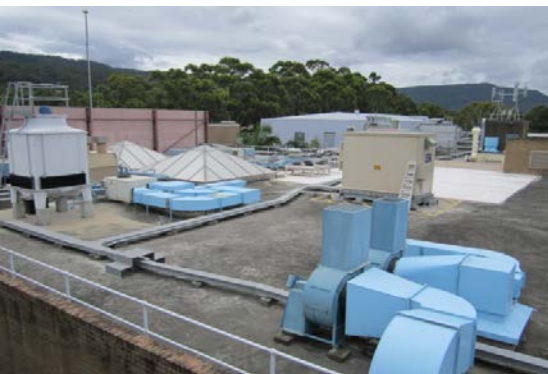
A/C vents and skylights
