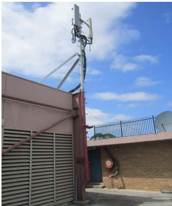
Telco Tower on Building 17 Roof - west
