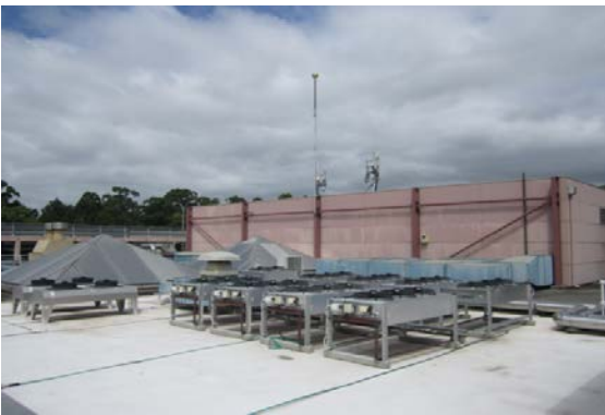
A/C vents and skylights
