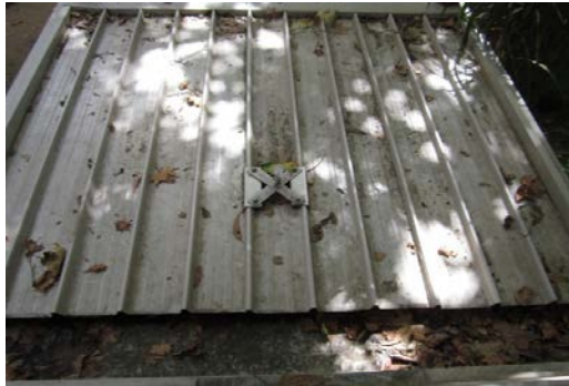
Anchor point on awning
