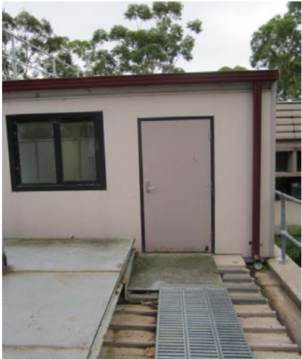
Walkway and access from door of plantroom
