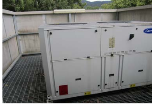
Enclosed landing and A/C Plant
