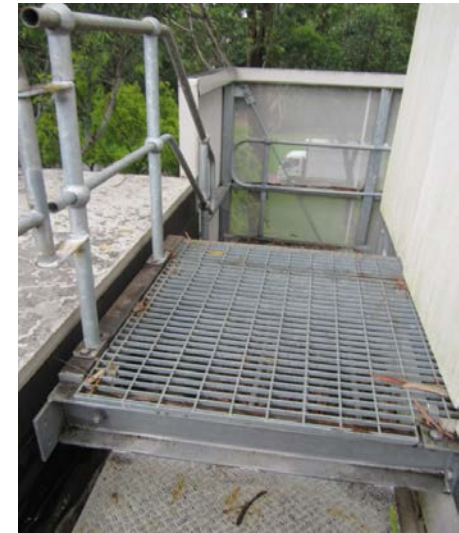
Steps up to landing and main plant
