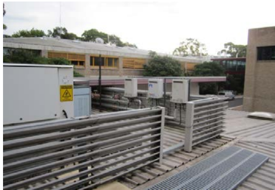
Enclosed services area
