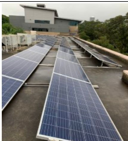
Building 3 roof area with solar panels installed caution when walking between rows
