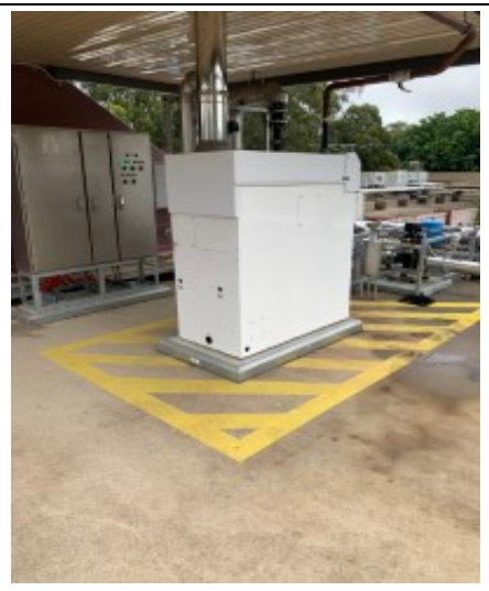
Building 3 roof area with chiller unit
