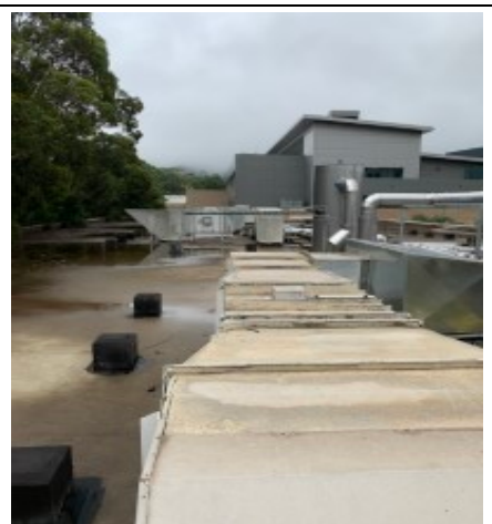
Building 3 roof area with ducts
