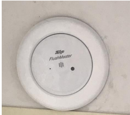
Figure 6: Automatic flushing system
