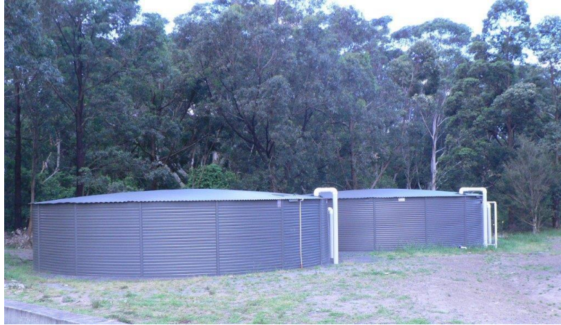
Figure 9: Rainwater Harvesting Tanks
