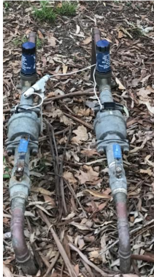
Figure 4: Water meters at UOW
