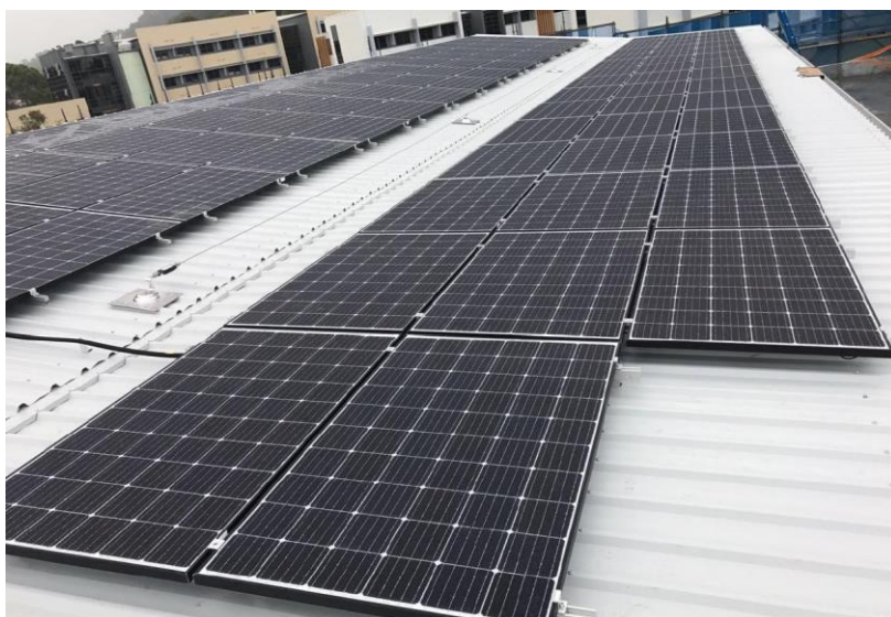
Figure 4: Solar PV System
