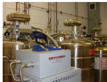
Liquid helium production plant.
